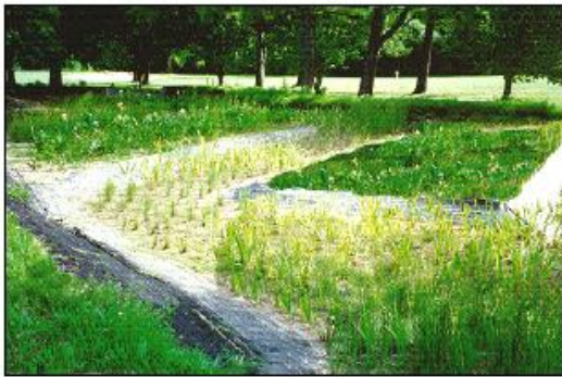
Newly Constructed Shallow Wetland
