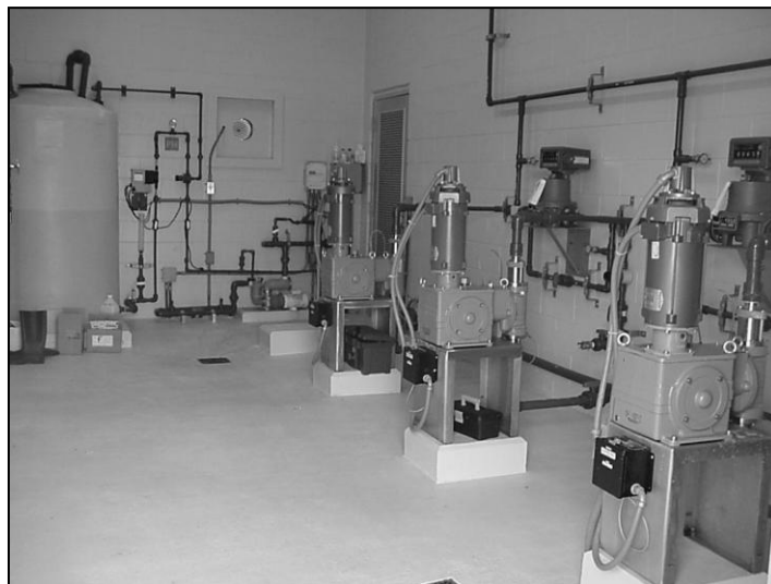
Figure 6.1 Alum Treatment System and Injection Equipment
